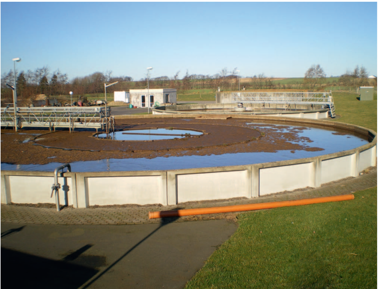
Figure 2. The biological process tank at Drøsbro is constructed as an annular shaped tank. Inflow to the tank takes place in the innermost ring to the anaerobic zone. From here the wastewater flows to the anoxic zone via an overflow weir before it via another overflow weir enters the aerobic zone in the outermost ring. Recirculation between the aerobic and anoxic zones is handled with a horizontal low head propeller pump.
